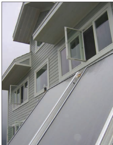
The Baxi solar panels blend nicely with the south-facing windows of the Kosmer home.
